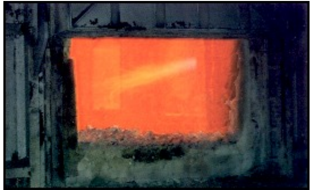
Furnace interior coated with ITC-100 and 296A
