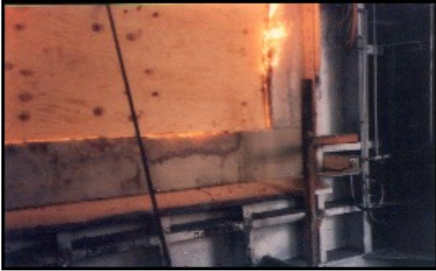
Plywood hot face coated with ITC-100 HT to enable emergency repairs of furnace door
